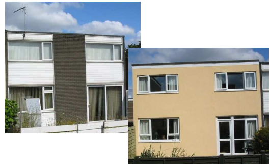
Refurbishment of Social Housing, Batemoor Close, Sheffield — £500,000 — Through-coloured insulated render system to approximately 150 houses.
